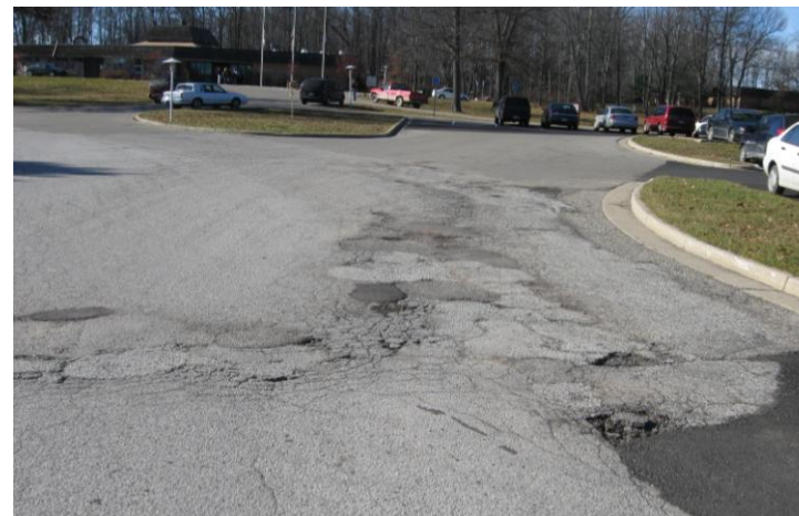
Deteriorated Parking Lots
