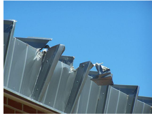
MTEC Roof repairs – damaged as result of ice buildup
